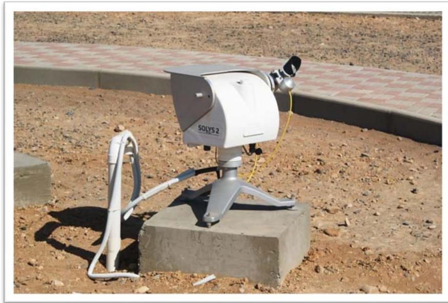
Figure 3-7: Sun Tracker with Pyrheliometer installed at Manah
